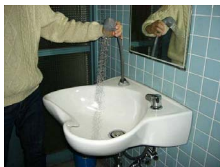
Emergency showers (located in washrooms)
