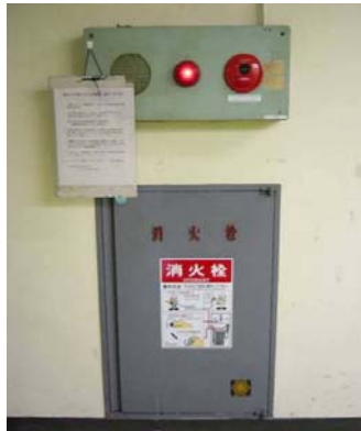
Fire alarm (top) and fire hydrant (below)
